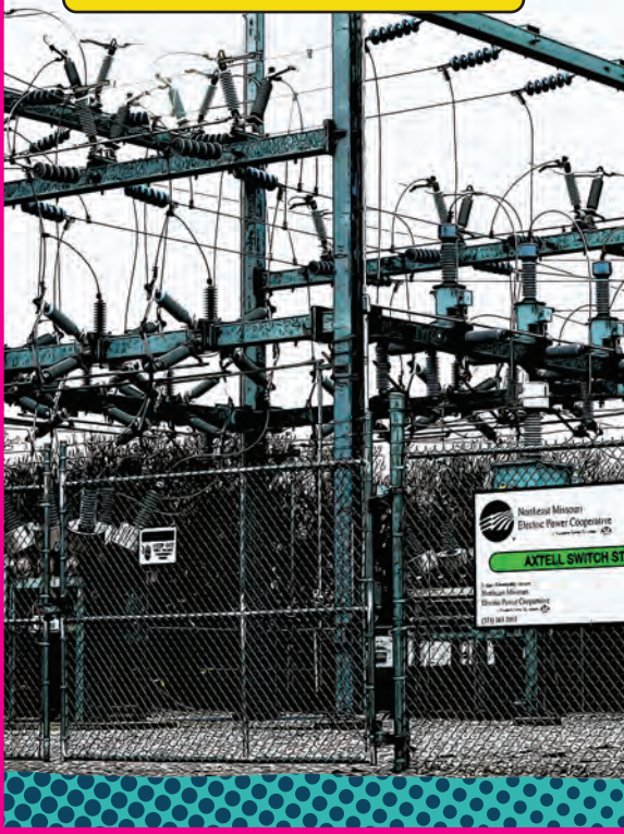
Axtell Switch Station completed in September 2023.
