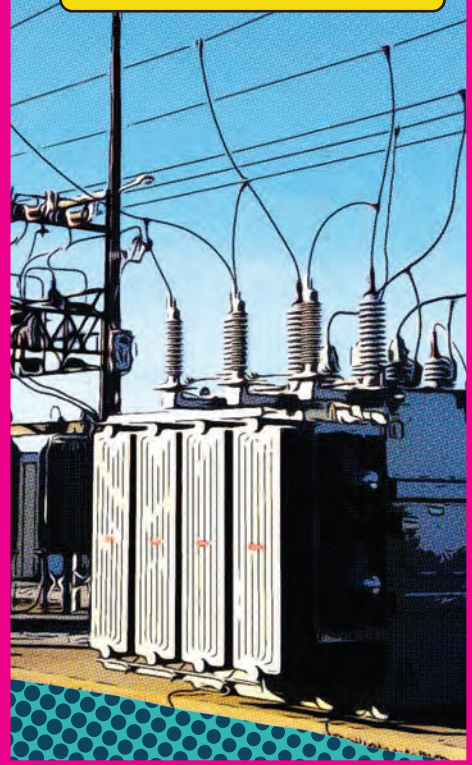
New transformer installed at Coppock Substation.
